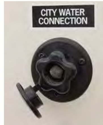
Typical city water fill connection
