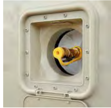
Typical external propane hook-up
