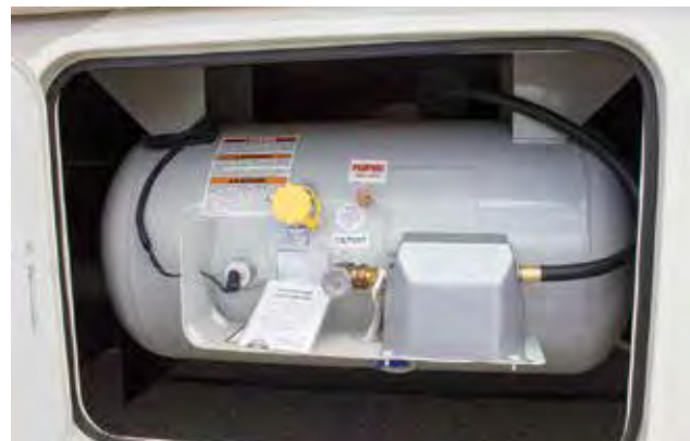
Typical propane gas tank
