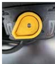
Safety Relay engaged, turning ON the battery pack
