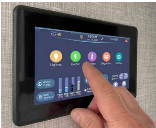
Typical Firefly Integrations multiplex main control panel. Features vary depending upon model and floor plan.
