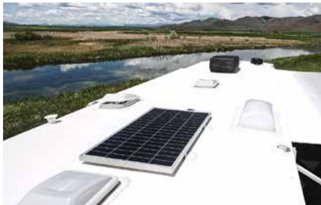
Typical Roof-mounted Solar Panel
