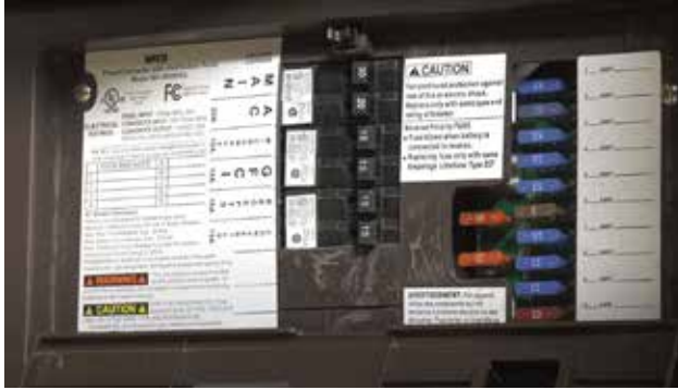
Typical 30-amp circuit breaker and fuse panel. Note circuit and device labels.
