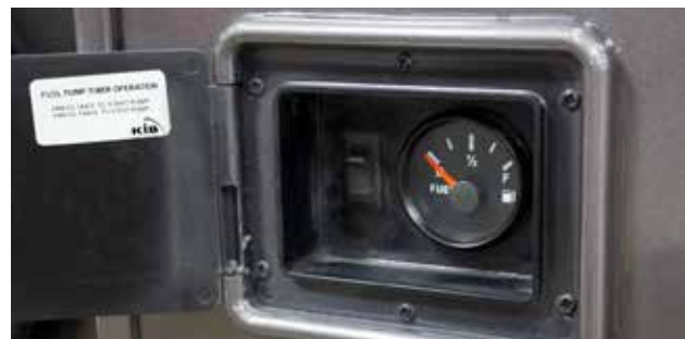
Fuel Pump Switch and Fuel Gauge for Fuel Transfer System
