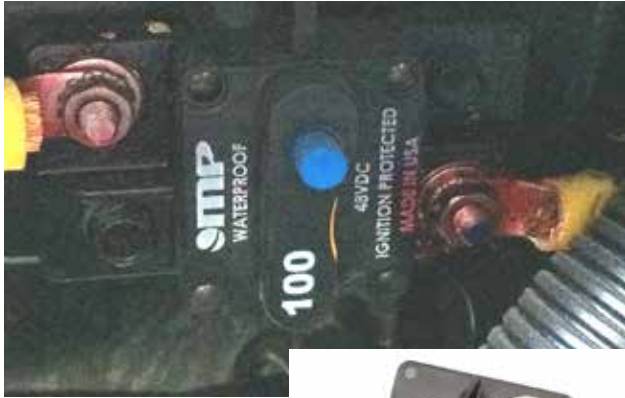
Typical Inverter Circuit Breaker located in the battery compartment.
