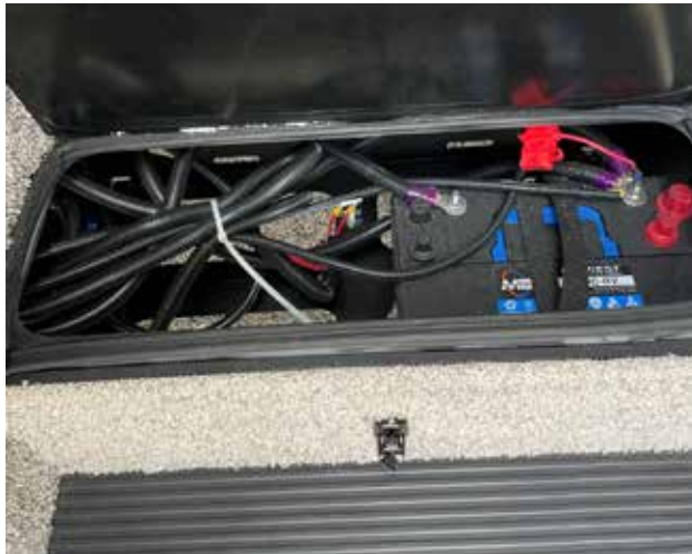
Typical Class C motorhome auxiliary battery location (under entrance step)
