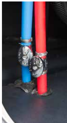
Typical low-point drain valves
