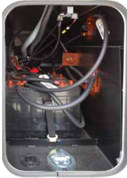
Typical Class A motorhome auxiliary (house) battery compartment
