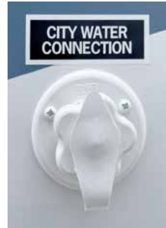
Typical city water fill connection
