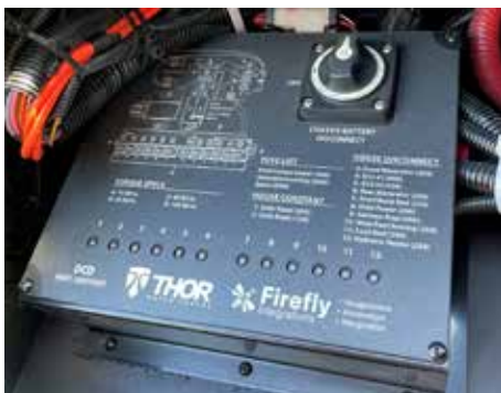
Master battery switch located on 12-volt circuit breaker panel.
