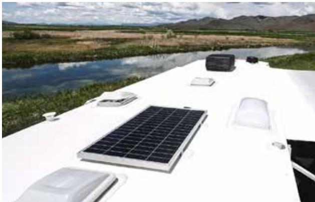
Typical Roof-mounted Solar Panel
