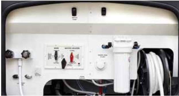
Water system panel for a Class A motorhome. Features vary by model and floor plan.
